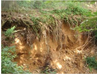
Storms are severely gouging out streambanks and sending sediment into Dyke Marsh. Photo by Glenda Booth
